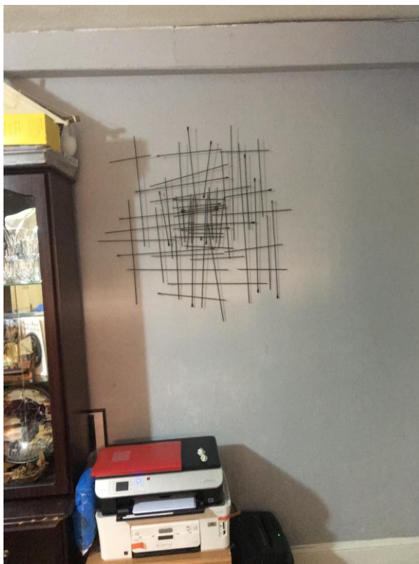
Slightly blotchy paint but no obvious cracks to ground floor rear reception
