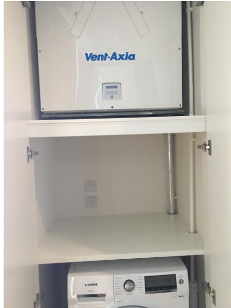
Utility Cupboard with Vent Axia Fresh air system
