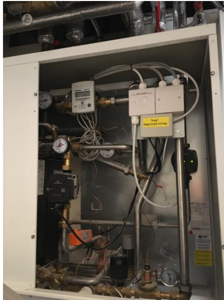
Hot water and central heating metered manifold from the communal boiler
