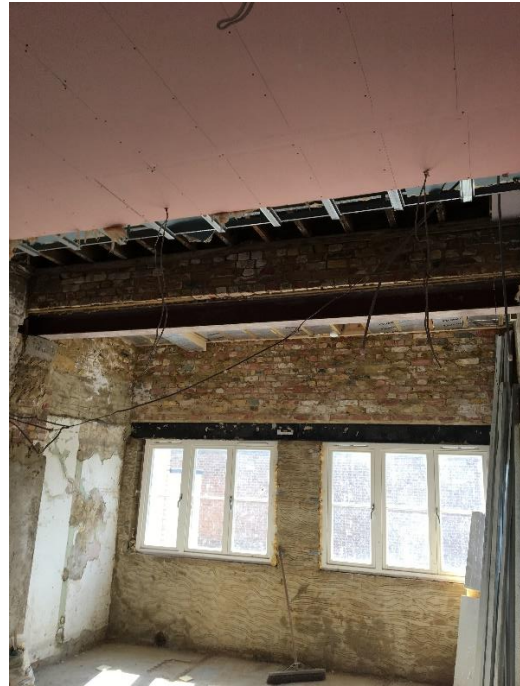
Incomplete Building Works
