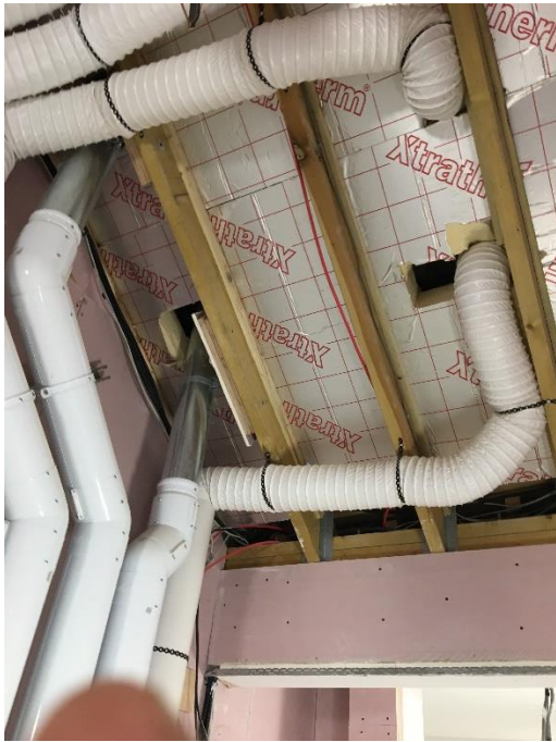
Incomplete Services Installation
