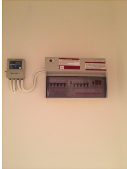
Modern Electrical Consumer unit, request a copy of installation certificate.
