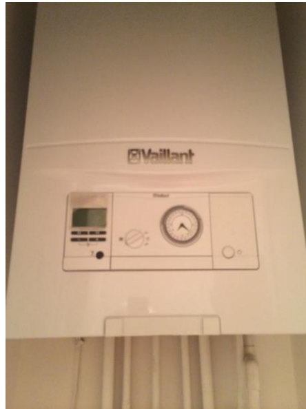
New boiler installed, request a copy of the installation certificate.
